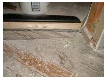
Layers, from bottom to top: Vib-X, 2x2" block, high-compression plywood, vinyl, plywood.
