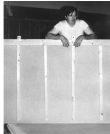
The author resting on a piece of a floating floor after installing polys. Alpha Audio Studios photo
